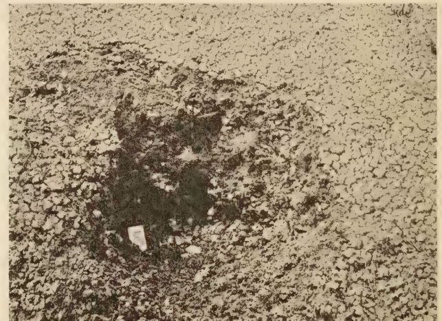
FIGURE 3.—RIGHT BANK AT STATION 105+16 SHOWING STRUCTURE OF LAYER 6 MATERIAL, AND SLOUGHED MATERIAL ON SURFACE
